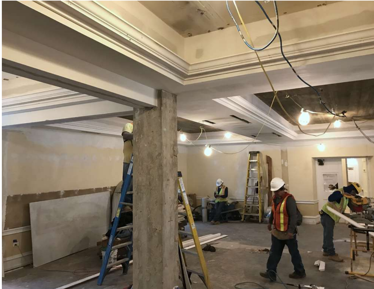
An electrician reworks fire alarm circuits, removes wiring for wall demolition, and installs electrical boxes for Assembly Room lights.
