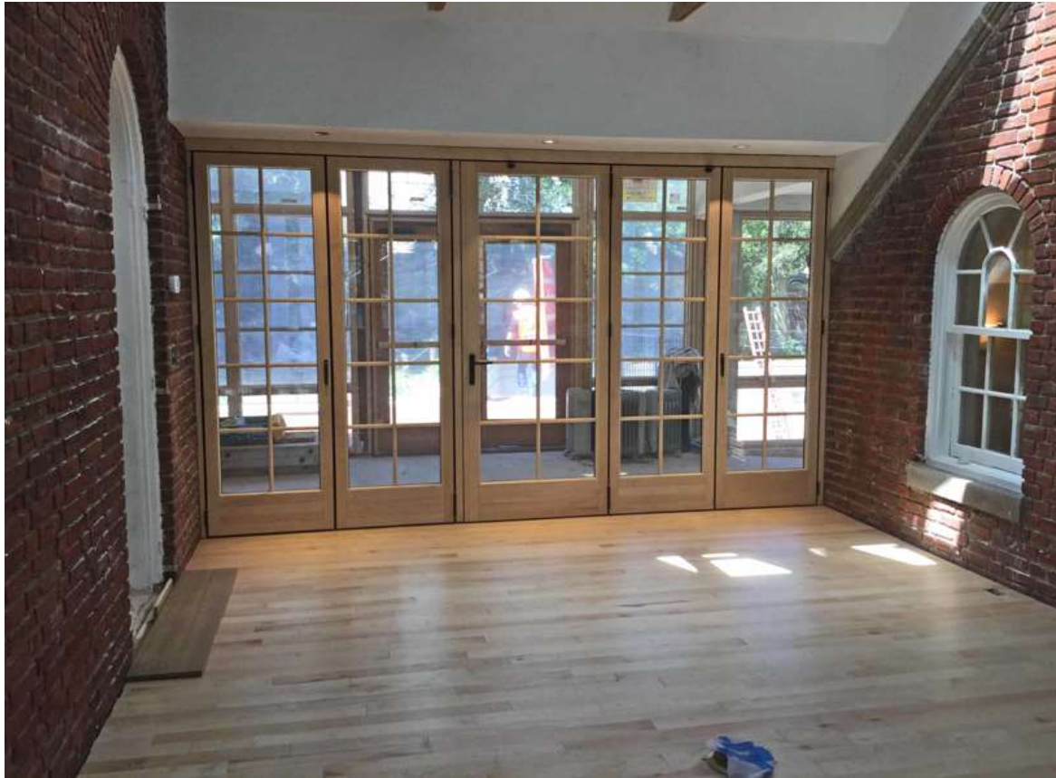
A flooring worker installs maple flooring in the new Carriage House room.
