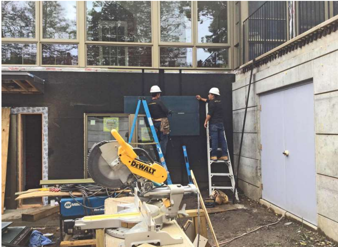
Arturo, Mario, and Douglas begin paneling the outside of the lower corridor.
