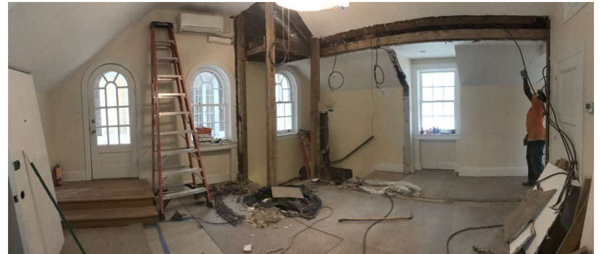
Tyrone and Tyrone and the electricians continue to remove walls to enlarge the Carriage House west office.
