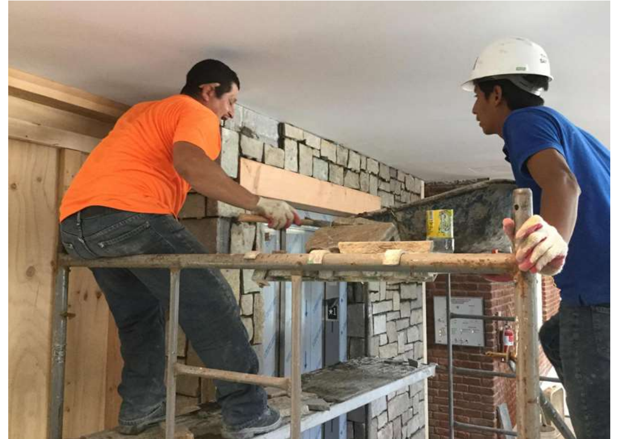
Two masons continue to install the elevator shaft stone on the ground floor.
