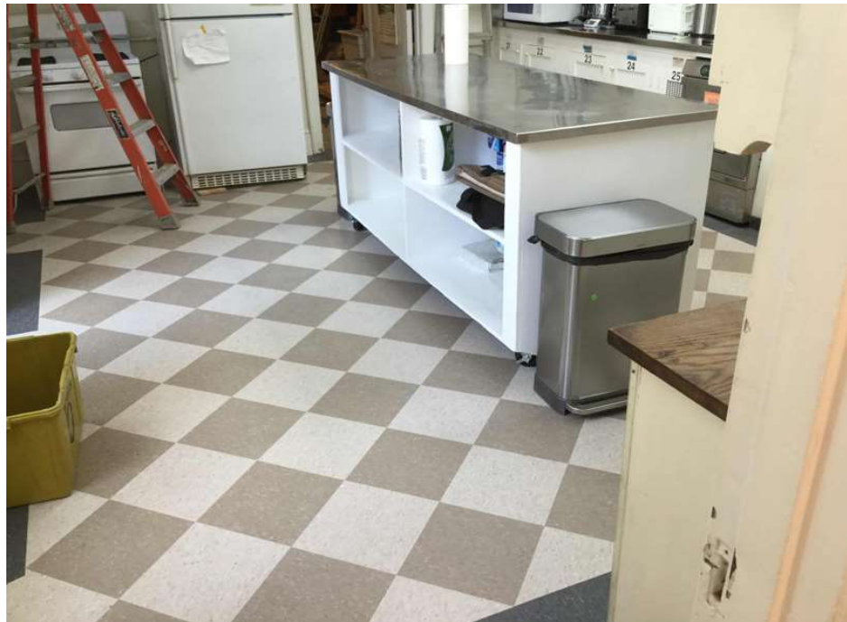
With new ceiling and floor in place, the kitchen is starting to look ready for duty.
