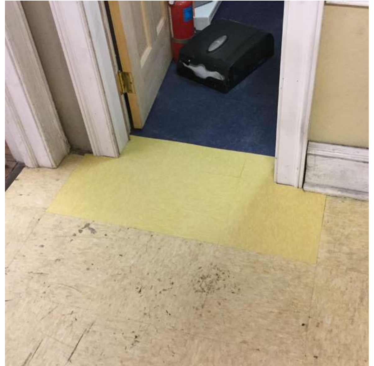
Tyrone patches the tile in front of the new Assembly Room bathroom door, but chooses a color a bit jauntier than the original.
